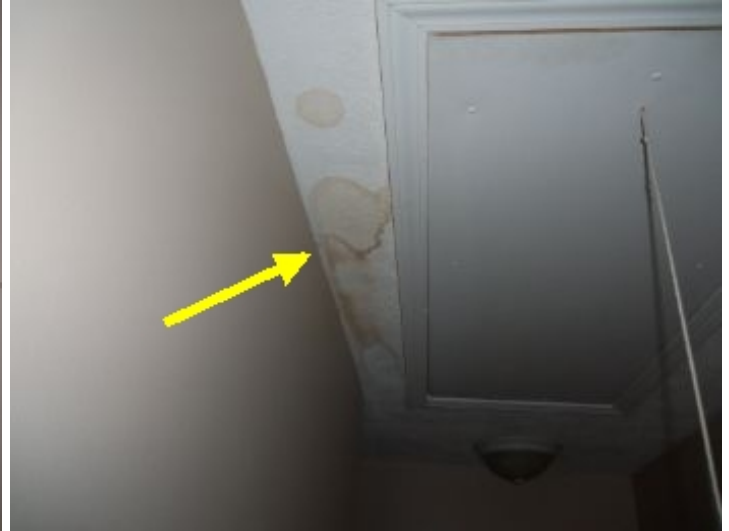
past water stain on ceiling by attic access
