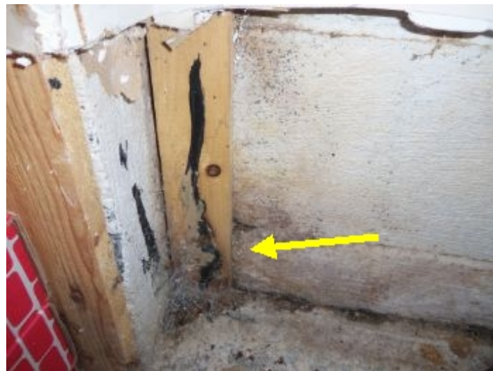
moisture damage to furring strip
