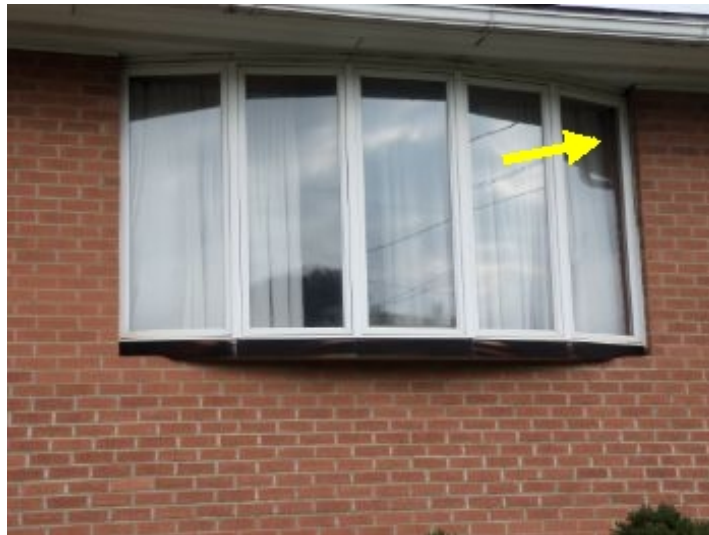
Bay window needs caulking repaired
