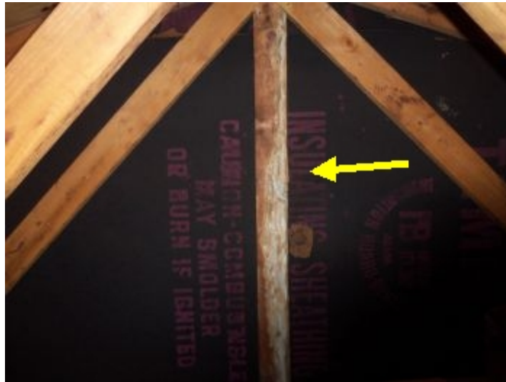
evidence of past water penetration
