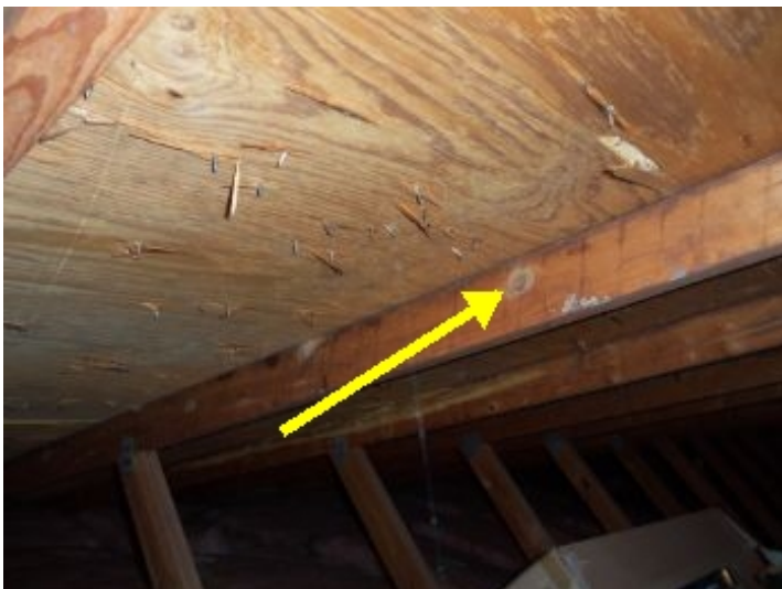
evidence of past water penetration
