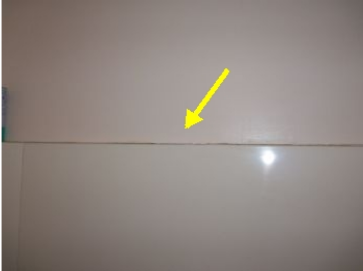
damaged caulking above shower
