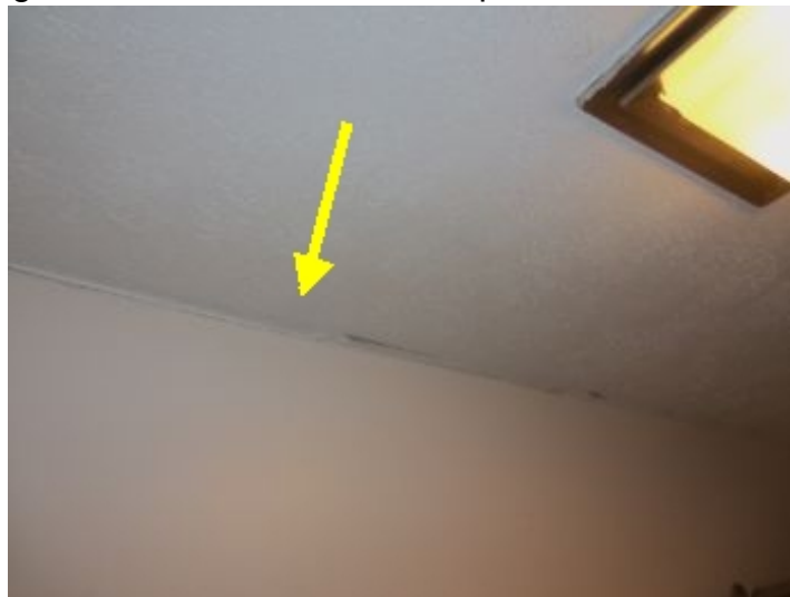
tape joint moisture damage
