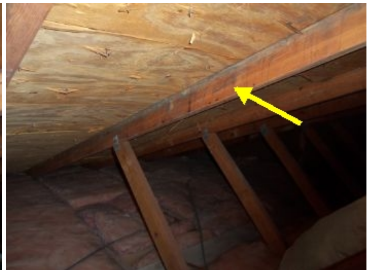
evidence of past water penetration
