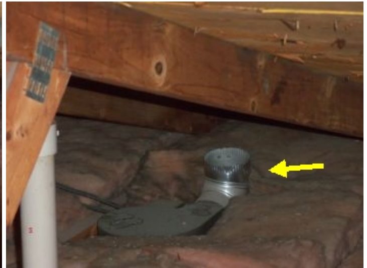
bathroom ventilation exhaust terminating in attic
