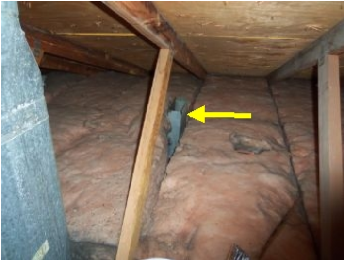
exhaust duct terminating in attic
